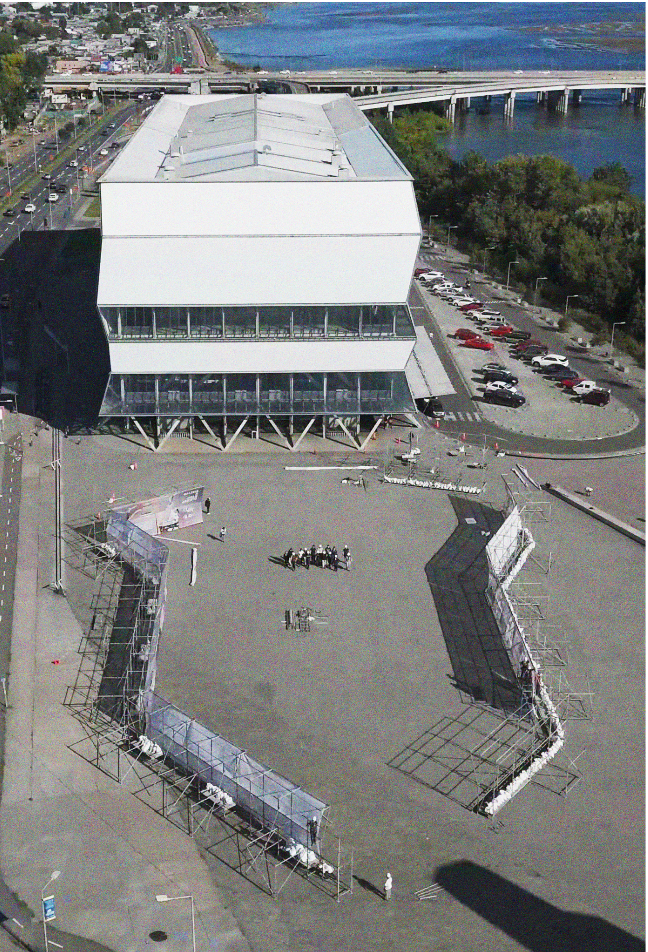
Aerial view of the pavilion under construction, with Teatro Biobío in the background
